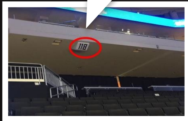
Custom Enclosure w/ Antennas Inside
