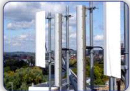
Mobile access, backhaul and packet core
